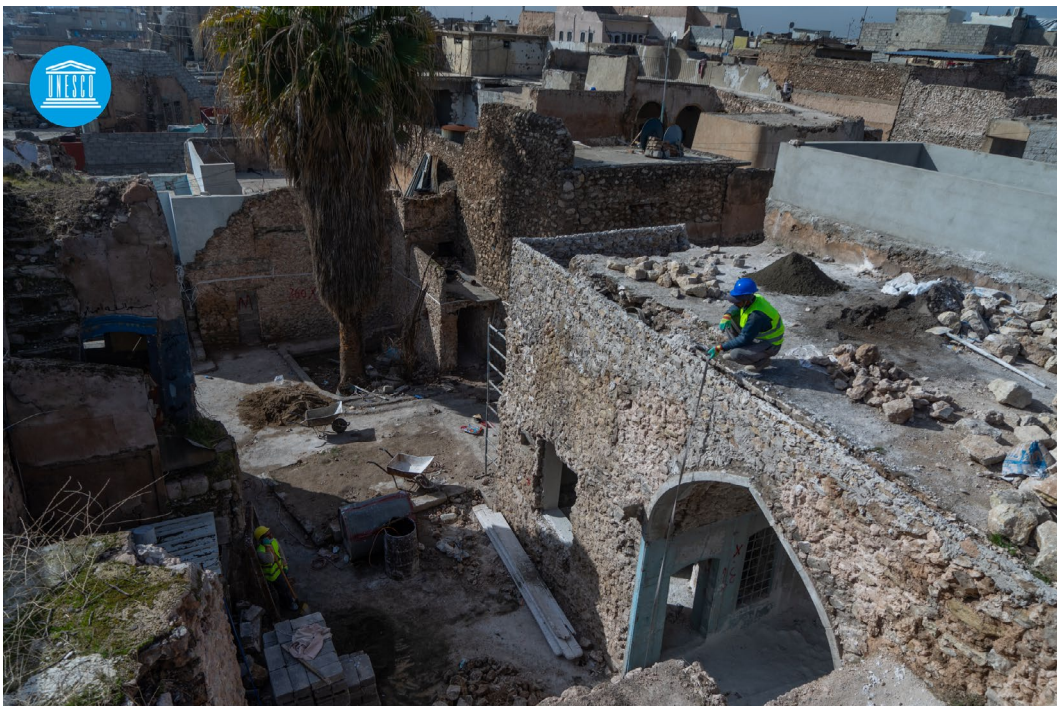
Culture and cultural heritage can have a major impact on a city's resilience: UNESCO's rehabilitation works in the Old City of Mosul, Iraq.
